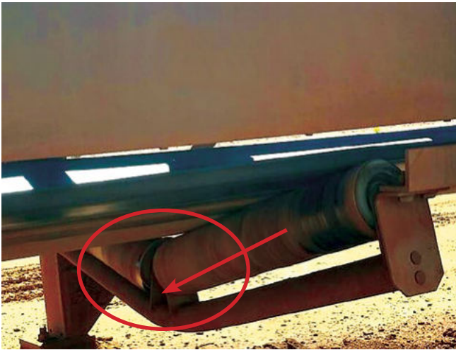
Idler Shell Collapse
